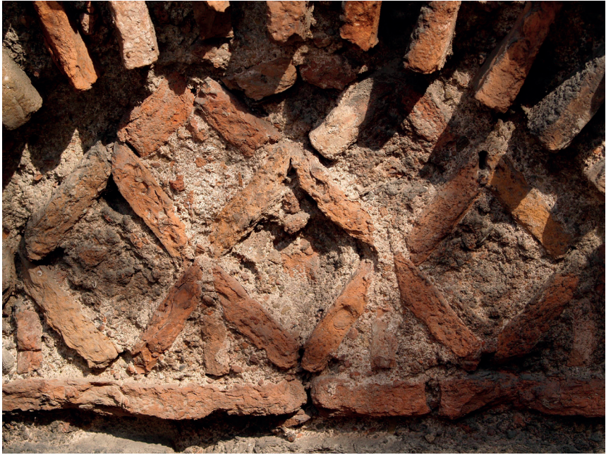
Figure 5a: Brickwork patterns. Bottom zone of the apse, Saint John the Baptist, Constantinople. Photo by Jasmina S. Ćirić.
