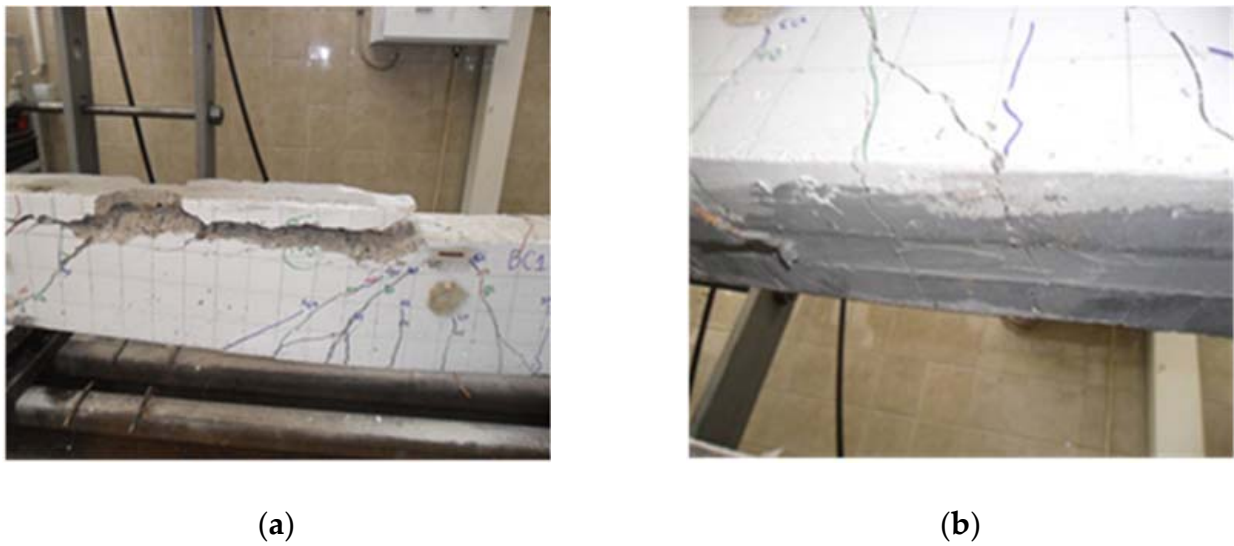
Figure 20. Beam B-C: (a) Concrete separation at the level of protective layer of concrete (b) Arrangement of cracks.
