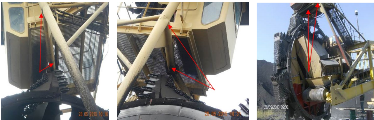
a) Right side of the structure, bent support and damaged welded joints
