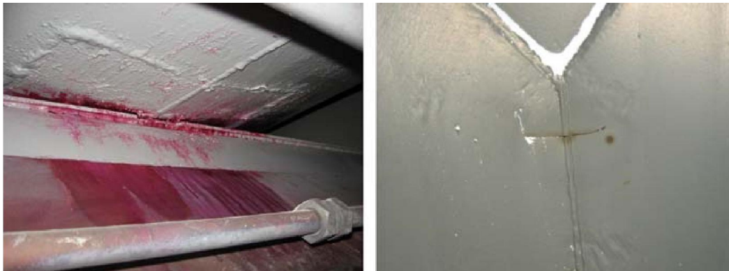
Sl.2 Observed cracks on the construction
