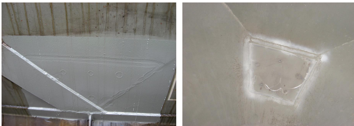
Figure 6. Crack repair on the tanks
