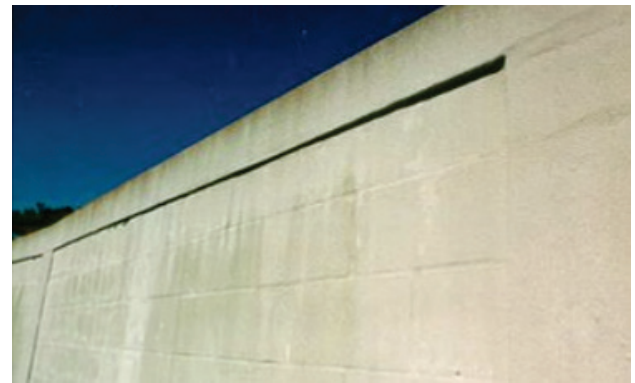
Figure 10. Sound barrier made of masonry blocks with Stucco texture [1]
