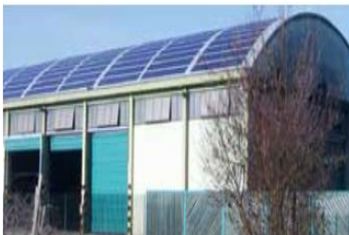
Figure 2. Flexible BIPVs - Thin-film solar plant on the arched roof of a waste sorting station in Monte Crocetta, near Vicenza (40 kWp), constructed in collaboration with Rewatt, Vicenza [7]
