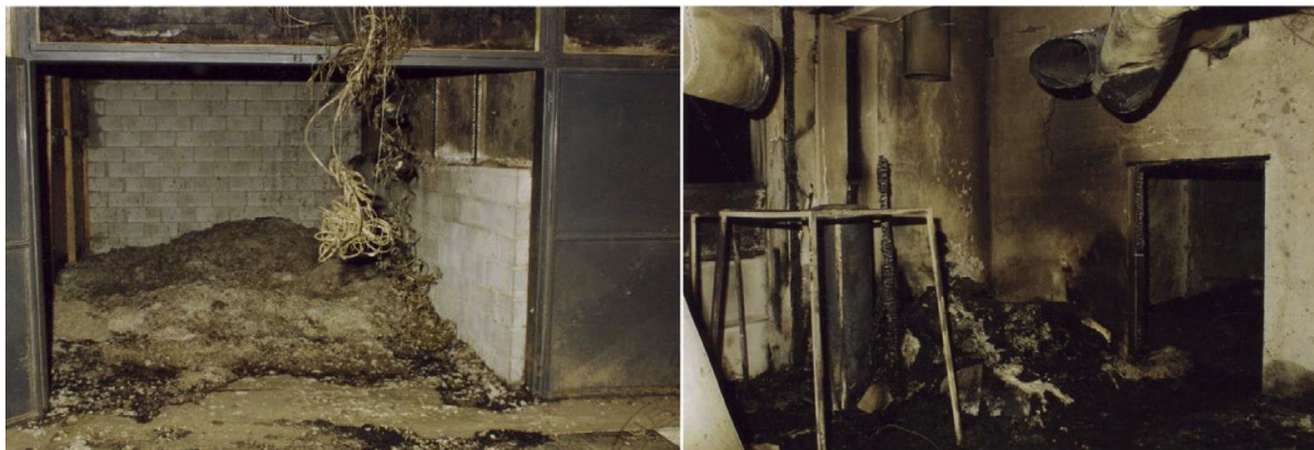
Fig.2 Textile industry facility after fire
