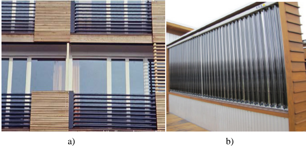
Fig. 3. Facade integration of evacuated tube collectors a) as balcony railings, Sunny Woods multi-family housing in Zurich, Switzerland, b) as fence in the driveway of the house, family house in Cyprus.
