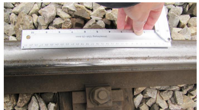
Fig. 4 Track condition on the measuring site
