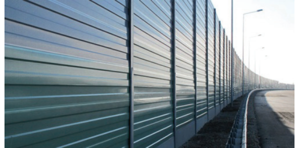
Fig 3. Metal noise barrier
