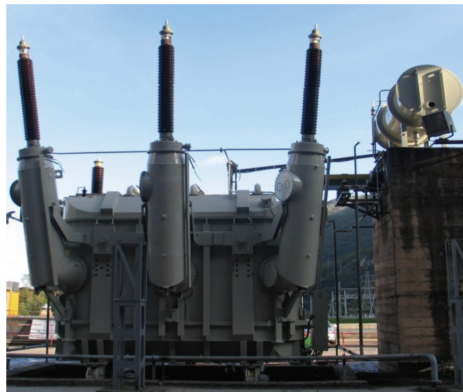
Fig. 1 Step up transformer 112 MVA
