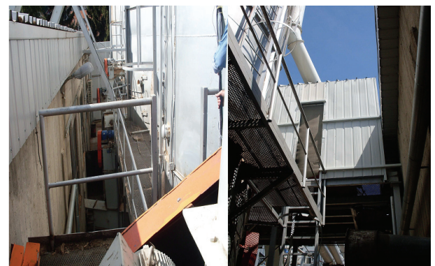
Fig. 11 Ventilator for extra drying of the chip – before and after sound protection
