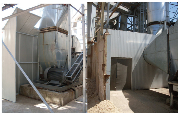
Fig. 8 Ventilator for chip drier with interlayer– after sound protection
