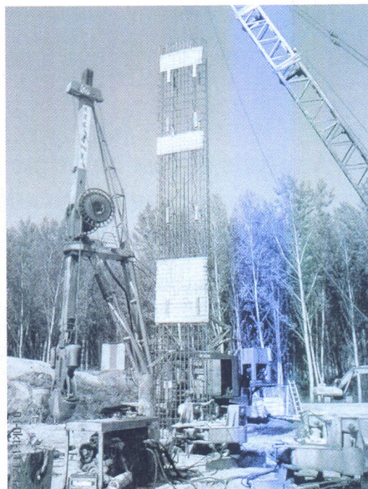
Figure 4: Installation of a reinforcing skeleton in a trench of a RC diaphragm
