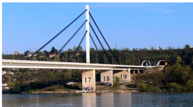
Figure 3. Landslide in the area of the Sloboda bridge in Novi Sad, with piers 17, 18, and 19 of the bridge.
