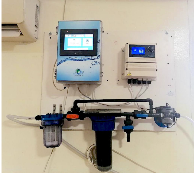
Figure 4. Device for measuring residual chlorine with automatic control and AI
