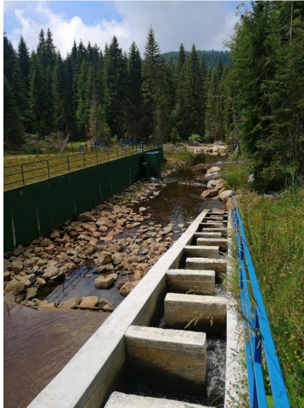
Figure 36. The small hydroelectric power plant on the Samokovska River (Kopaonik National Park). This river is the largest in the National Park and had a sustainable population of brown trout until the small hydroelectric power plant was constructed. The river's upper course has also been affected by organic pollution from the wastewater of the winter tourist complex (photo by V. Simić).
