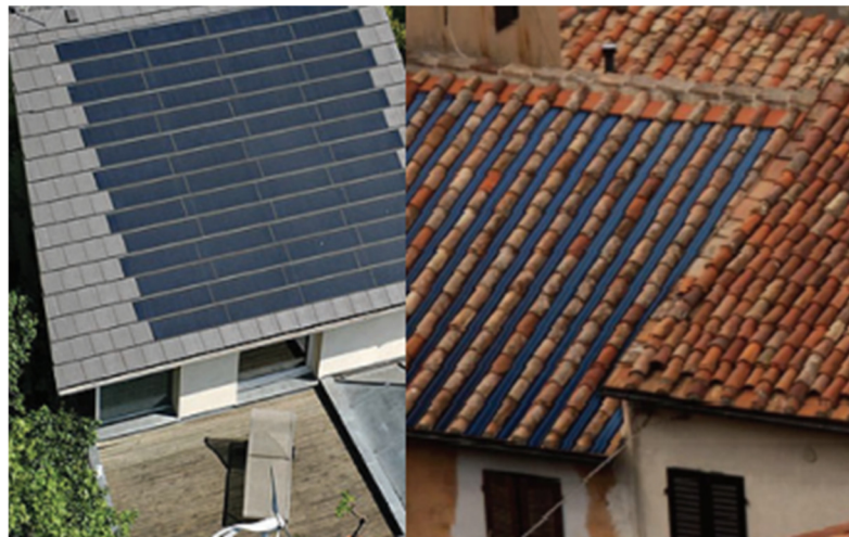
Figure 6: Examples of BIPV installation on roofs [24]
