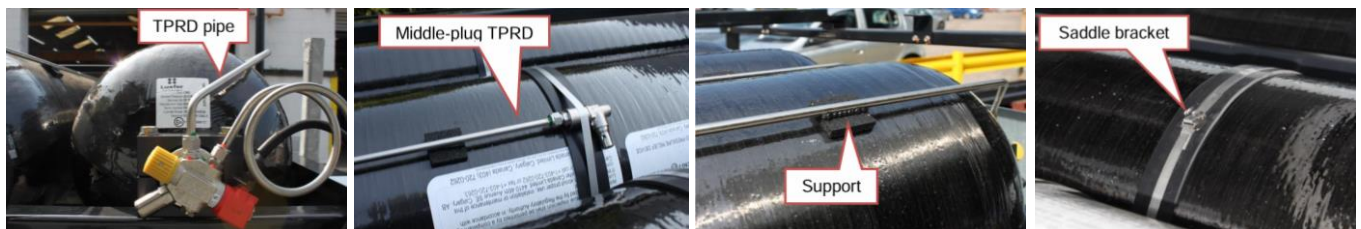
Figure 4 TPRD Pipe, Middle Plug and Saddle Bracket on Bus-Mounted Cylinders
