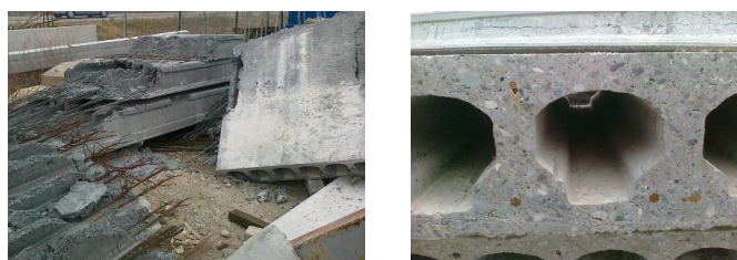
Figure 1. Mechanically damaged hollow-core slabs.
