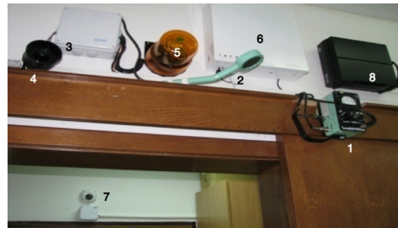
Figure 2. Our alarm system
